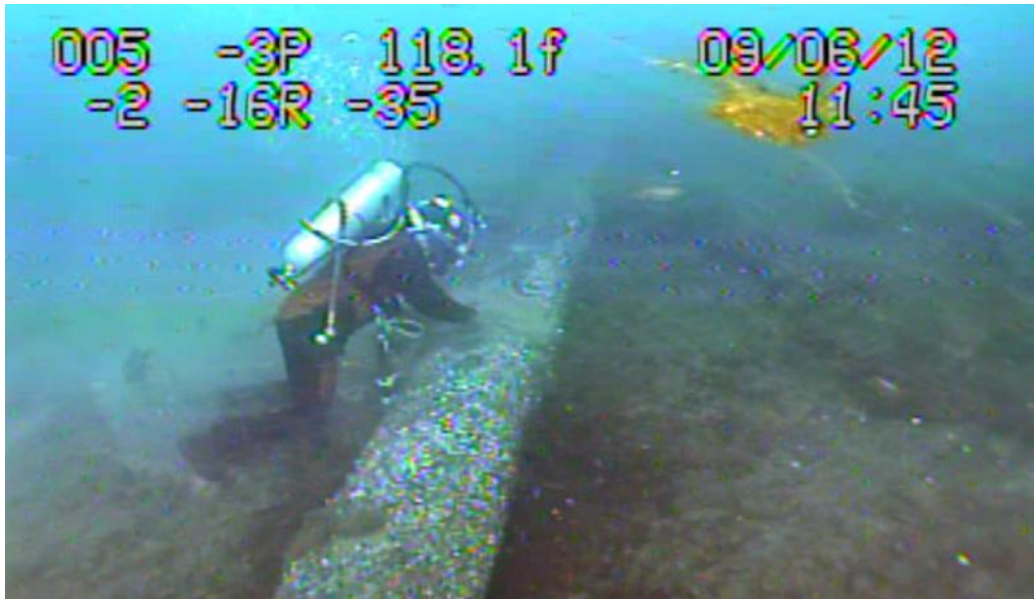
Figure 5 – “A diver inspects Enbridge's Line 5 pipeline under the Straits of Mackinac for a possible dent.” 23
